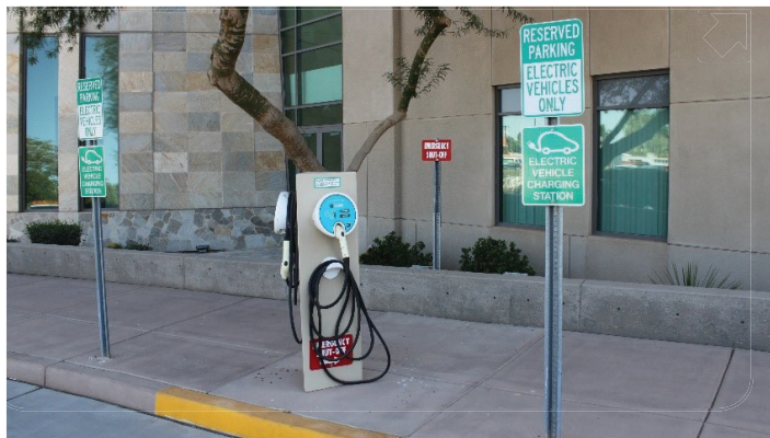
Electric Vehicle Charging Station (Source: Yuma County Airport Authority)
