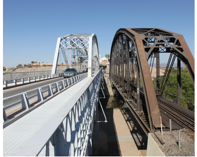
Ocean-to-Ocean Bridge and Union Pacific Railroad Bridge over the Colorado River (Source: Kimley-Horn)
